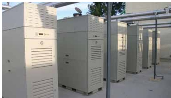
Six Capstone microturbines provide heating and onsite power at this Southern California college.
