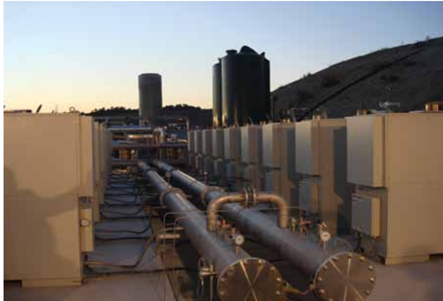
Eighteen C65 microturbines running on methane gas generate power and heat at Mentaure Landfill in France.
