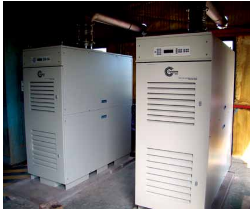
Eleven Capstone C65 natural-gas microturbines power compressors at this Bolivian pumping station.
