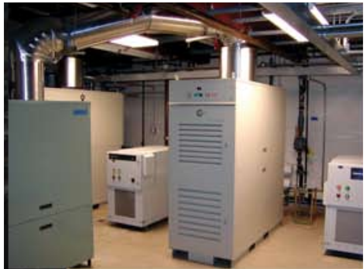
Capstone microturbines generate electricity, cooling, and heating at Vineyard 29 in Napa Valley, California.
