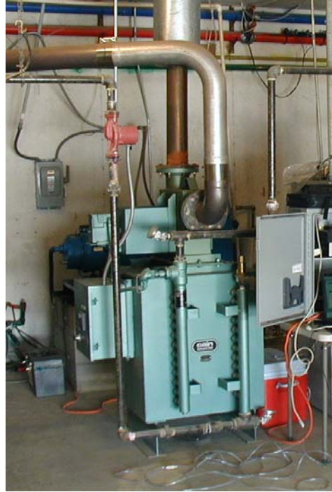
Cain Industries Heat Recovery System
